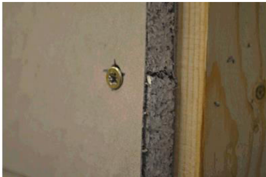
Figure 34 Breathaboard Localised Splitting Failure
