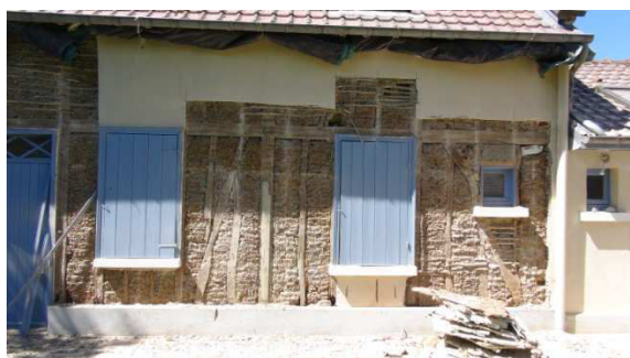
Fig. 5: Removal operation of the coating of cement and the wattle and daub
