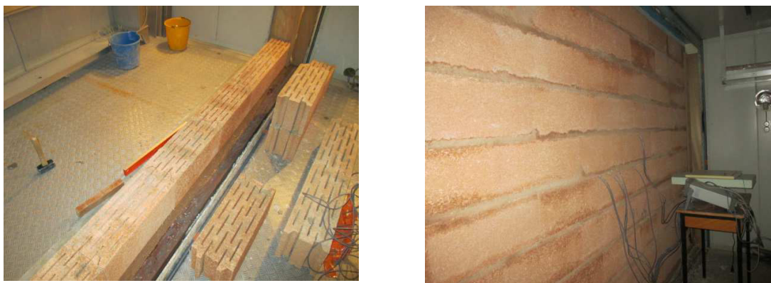
Fig. 7. Photographs of the construction of the wall between the two chambers (on the left) and of the sensor wires going out of the wall in the hot chamber (on the right).
