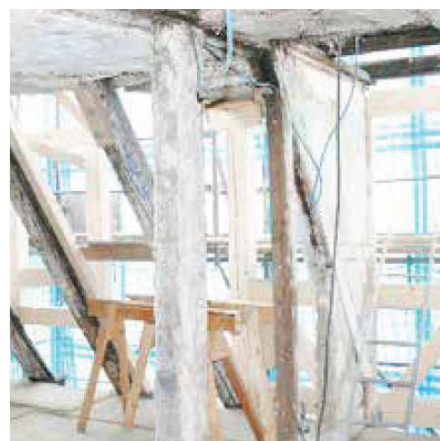
Fig. 6 Condition of the wooden framework before restoration, picture by Alexandra Fritsch.
