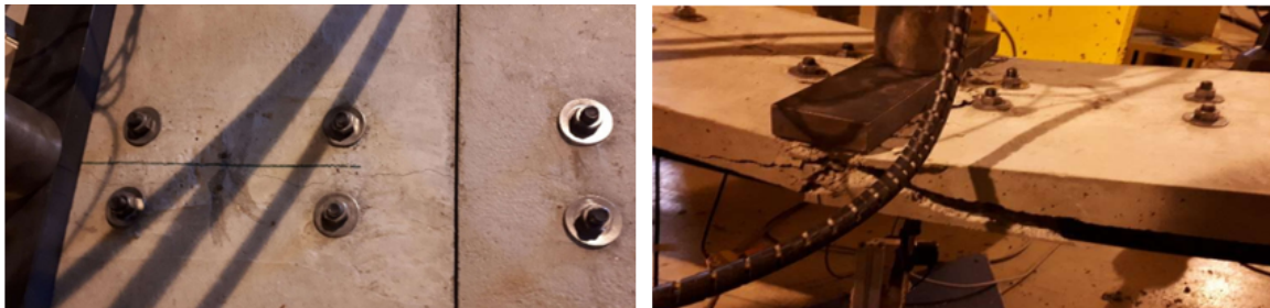
FIGURE 10. Cracks between bolt rows and crushing of the intermediate concrete block
