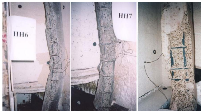
Figure 1. Spalling in HPC columns ( Benmarce and Guenfoud, 2005).
